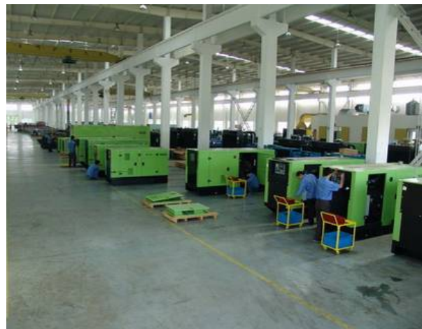
Workshop of silent generator set
