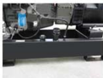
Base Fuel Tank
